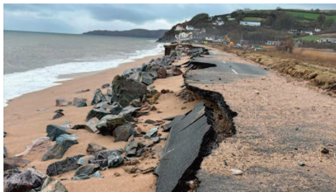
The A379 has been severely damaged on this coastal section. (Image: Devon County Council)
