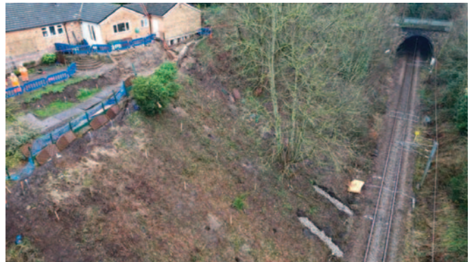
The same spot as the previous picture, this time after days of heavy moving have taken place. (Image: Network Rail)
