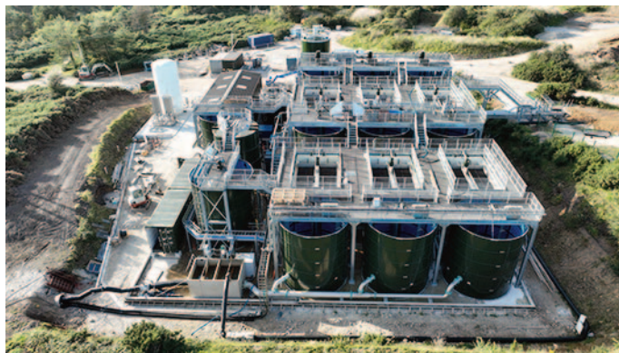
The newly built plant that is purifying the mine waters being pumped from South Crofty. (Image: Cornish Metals)
