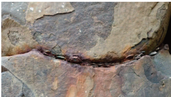
The coins have been placed into joints within the basalt columns and are now expanding as they rust. (Image: National Trust)
