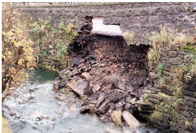
Part of the collapsed retaining wall at Brough Bridge. (Image: Derbyshire County Council)
